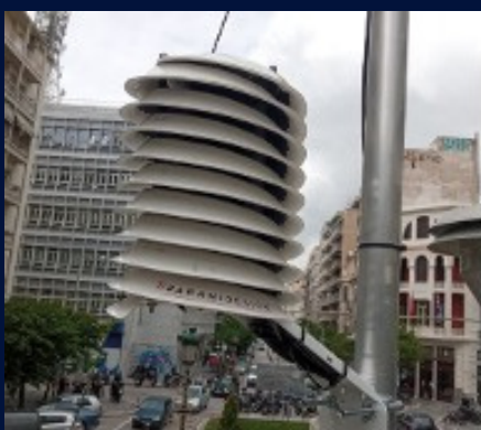
Barani weather station installed in Thessaloniki
